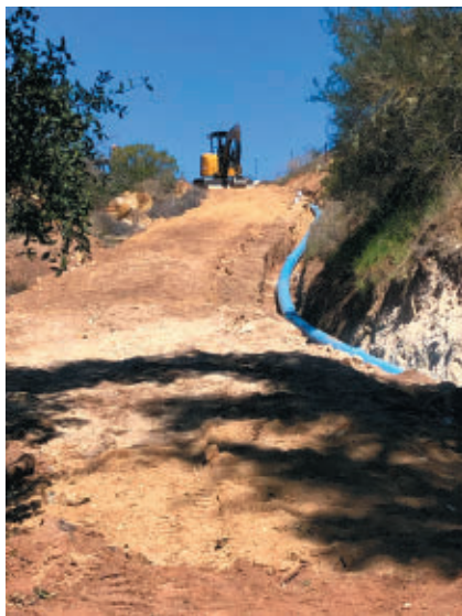
The construction of the upsized waterline to deliver water from the existing pond near the entrance to the large pond by the shop.
