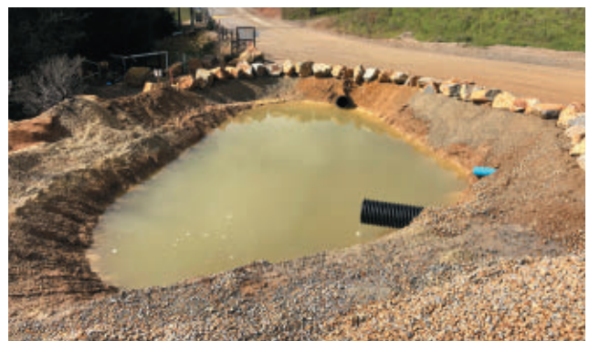
The new pond was constructed to slow water flowing into the existing primary stormwater pond near the plant entrance.
